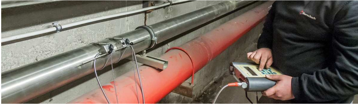
Figure 2 mobile ultrasonic flow measuring. 11
