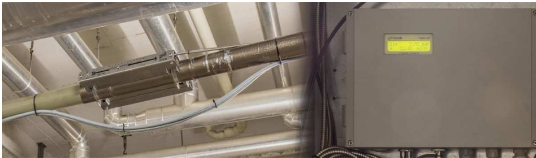
Figure 3 Stationary flow monitor with installed ultrasonic clamp-on sensors. The silver layer is damping material to avoid reflections and noise from the pipe. 12
